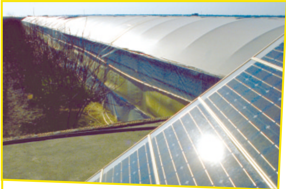
Solar Photovoltaic installation for green house water irrigation
